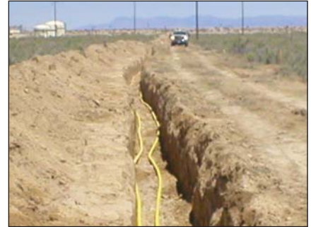
Figure 3: Questar Gas installed about 4,200 feet of PA-11 pipe as two parallel 2-inch SDR11 pipelines serving a single industrial customer and operating at 200 psig.
