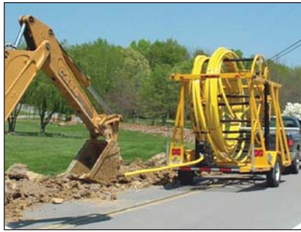
Figure 2: A backhoe was used to pull the pipe from the unwind stand, through the straightener, and off the trailer.
