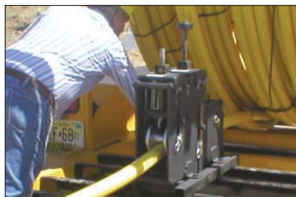
Figure 1: PA-11 pipe uses conventional straightening and re-rounding tools. One end of the pipe was directed through the straightener and secured to a cable.
