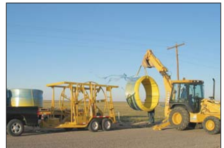
Figure 4: Loading a 1,000-ft coil onto the PLCS deployment trailer for the PNM installation.
