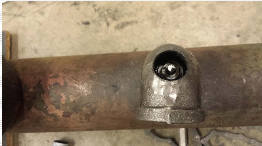
The operation is complete. Rubber stopper inserted into the elbow. Equipment removed. Elbow can be removed from the main and abandoned according to company procedures.
