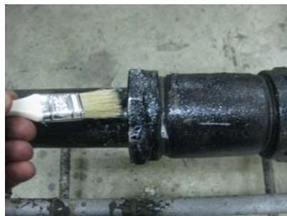
Soap test again to make sure no leaks were caused by blasting.
