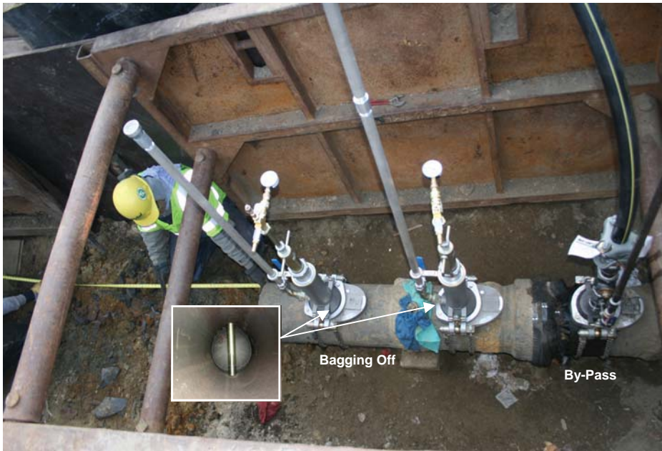
By-Pass Assembly and Bagging Off System for Gas Flow Stopping Shown
