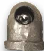
Top view: Hole drilled and rubber plug inserted to stop the flow of gas.
