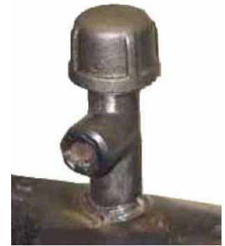
3/4"-1 1/4" Mueller Tees Missing the Completion Plug.
